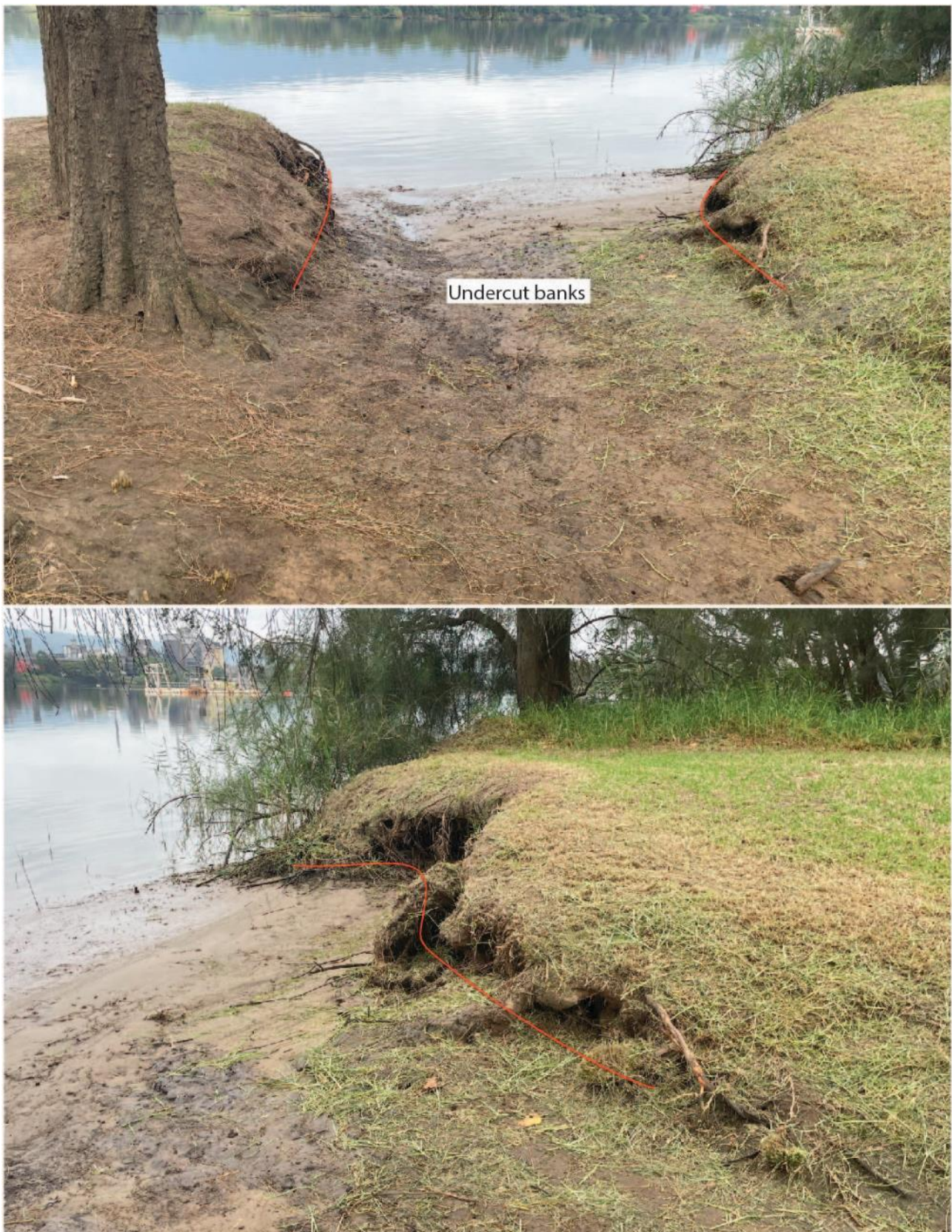
Figure 7-3 Stormwater outlet eroding at riverbank
