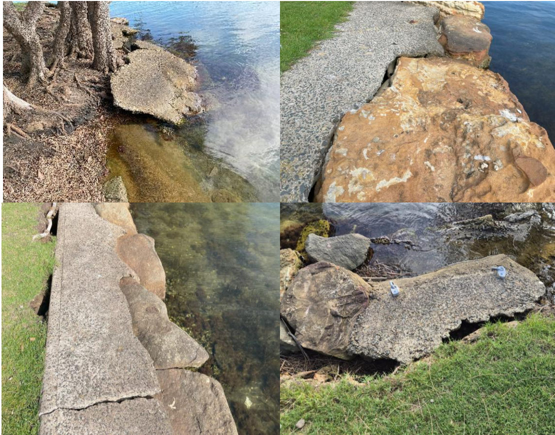
Figure 3-6 Examples of concrete reinforcement in poor conditions
