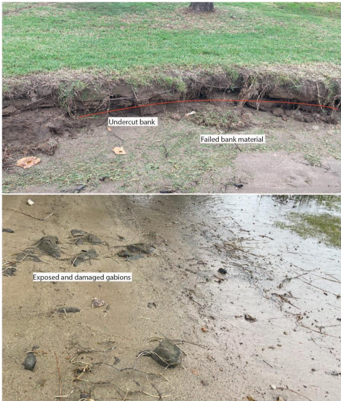
Figure 7-2 Eroding bank at the beach, with partially exposed gabions
