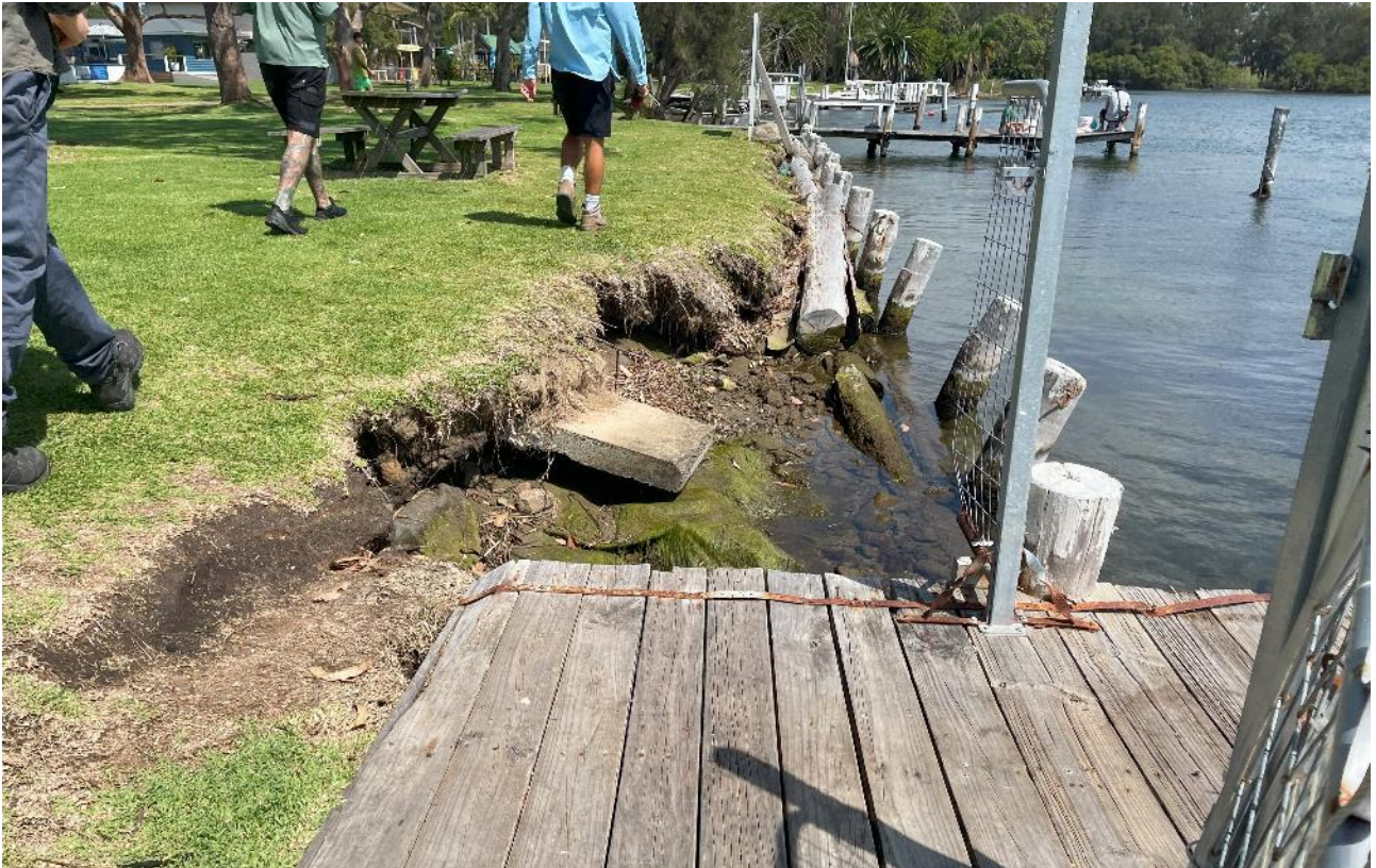
Figure 5-5 Foreshore erosion and failed log revetment
