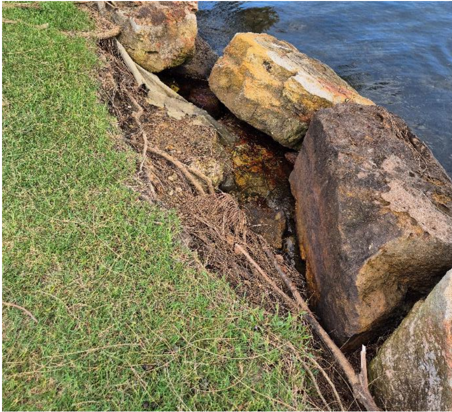
Figure 3-7 Rocks collapsed into the lake
