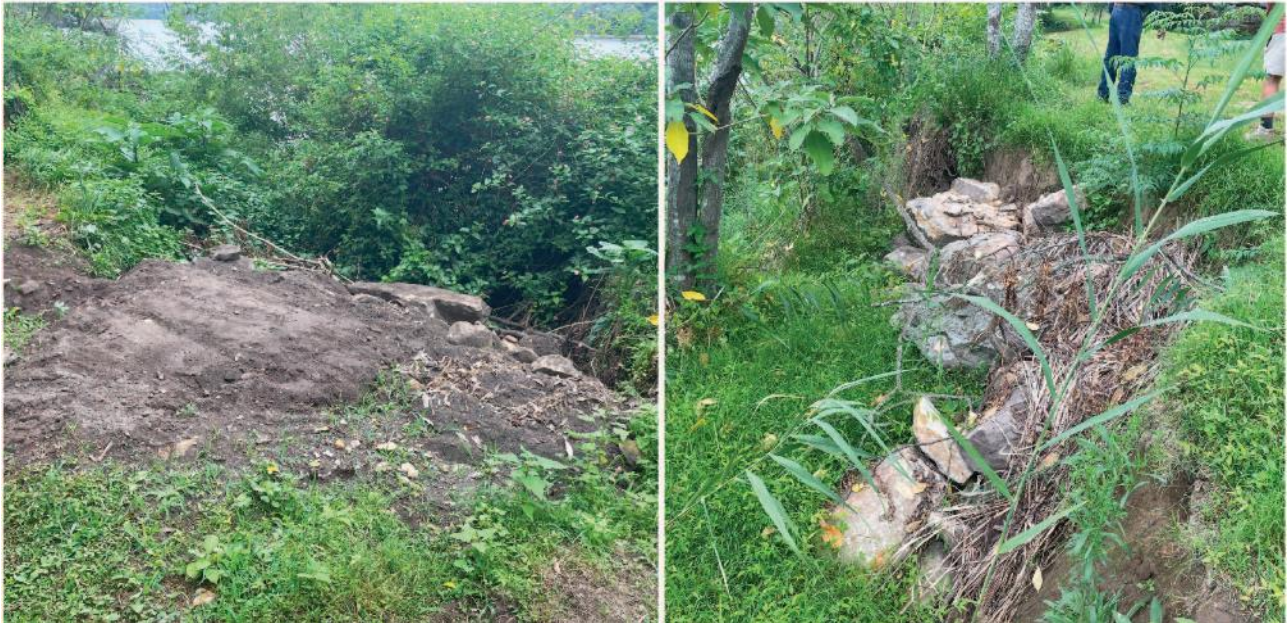
Figure 4-3 Informal works to treat erosion.
