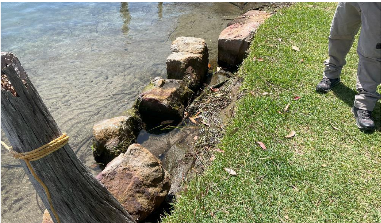
Figure 5-4 Rock beaching undermined and collapsed into the water
