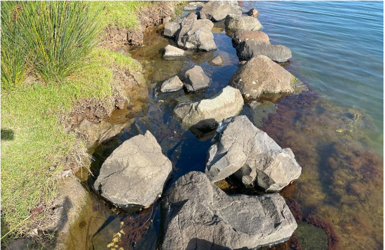
Figure 3-4 Ineffective Foreshore Rock Protection
