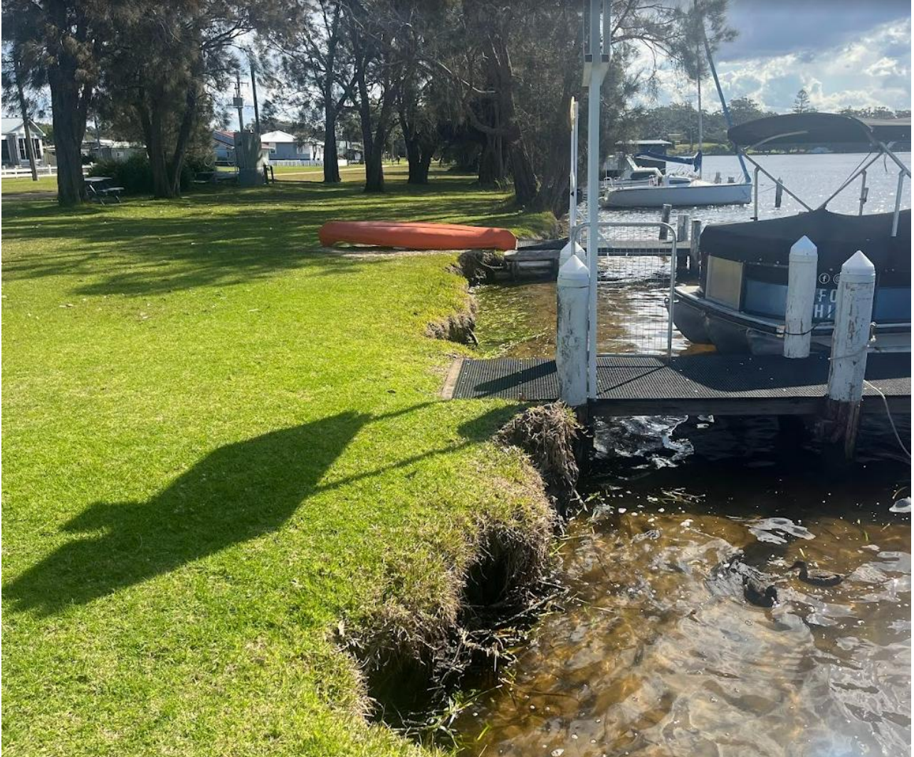
Photo 1: Foreshore showing evidence of erosion. Also showing commercial jetty structures
