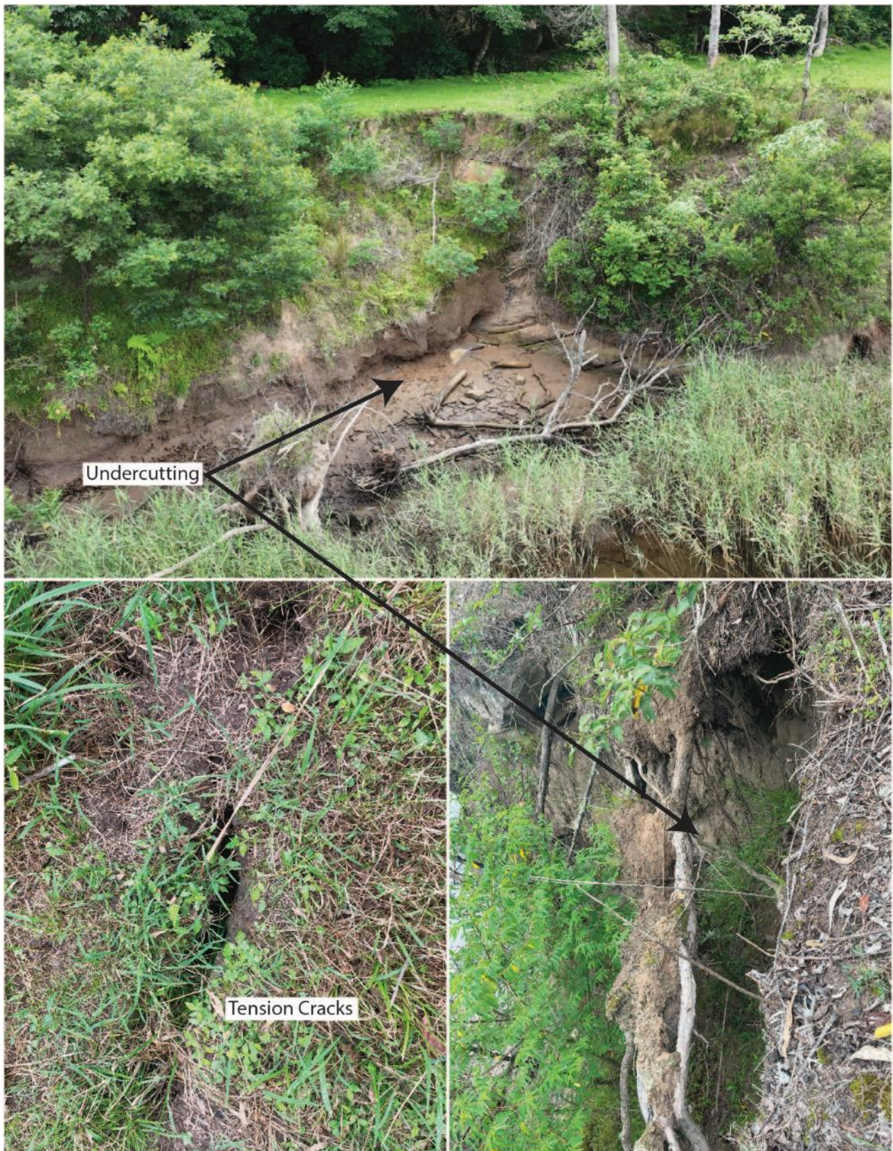
Figure 4-2 Undercutting of the bank captured by the drone and from the bank. Tension cracks in the top of the bank viewed from above.
