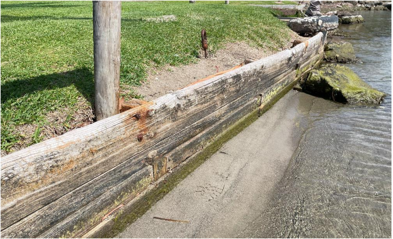
Figure 5-7 Scouring behind wood revetment
